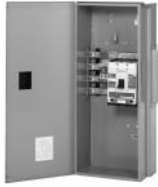
Main Circuit Breaker
