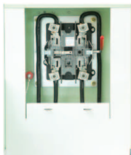
Bypass Section—Test Block
